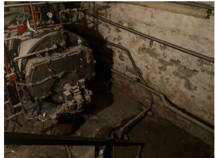
12 Boiler and sump observed inside 435 Wales Avenue.
