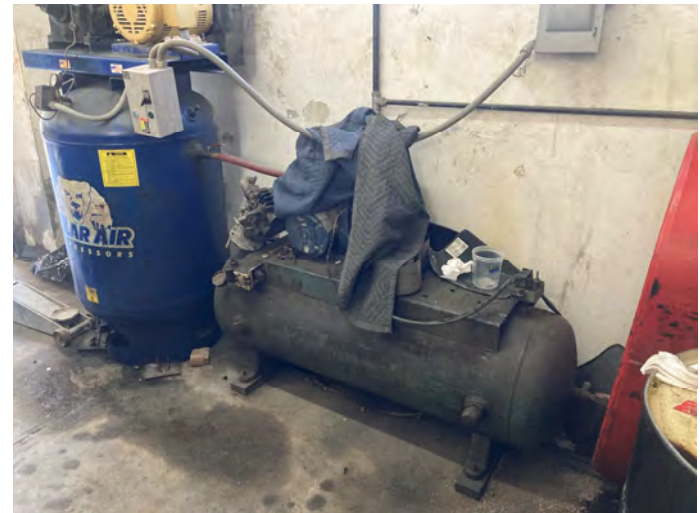
04 Two large air compressors inside the 435 Wales Avenue garage with staining present on the concrete floor.
