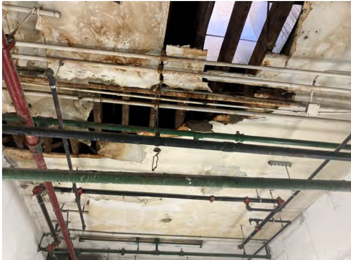
15 Ceiling and water damage inside 435 Wales Avenue.
