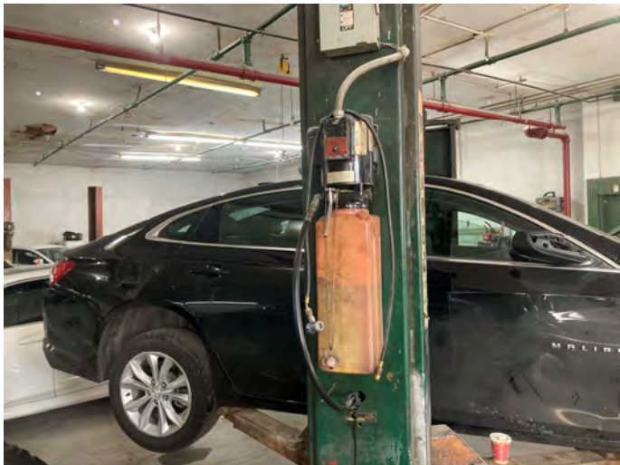
11 Hydraulic fluid container mounted on the side of a hydraulically operated vehicle lift inside 435 Wales Avenue.
