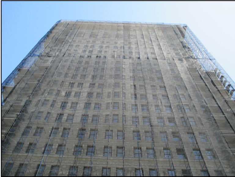
3. View of the Project Area looking southeast from the west side of Fifth Avenue.
